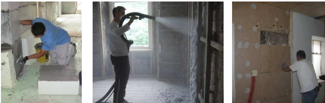
Figure 1: left: installation of internal insulation (Perlite) at Villa Castelli © Eurac; middle: Blowing on the wet cellulose insulation material © HES; right: installation of wood fibre © Eurac
